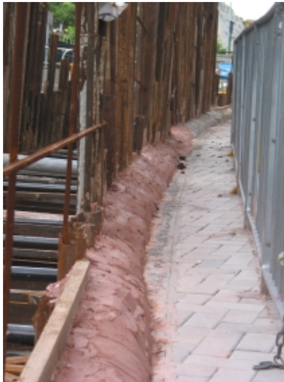
Plate B4 – Sheet piles protruding above ground with cement mortar wedge applied to prevent surface runoff
