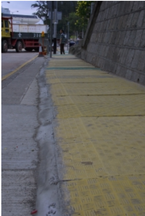
Plate B2 – Typical pedestrian crossing trench opening which is also effective for preventing surface runoff and infiltration of rainwater
